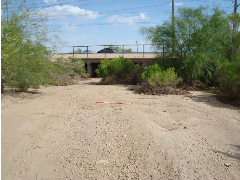
Photo 2. Wash 1 (W1) facing south (downstream) toward Pecos Road; 4-foot-long scale
