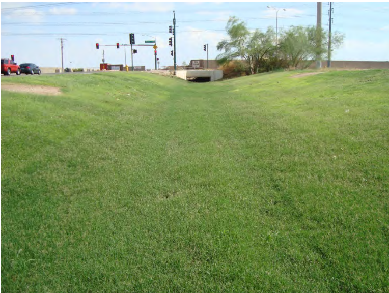
Photo 7. Constructed channel 2 (C2) along 32 nd Street facing south (downstream) toward Pecos Road; provides stormwater drainage for development
