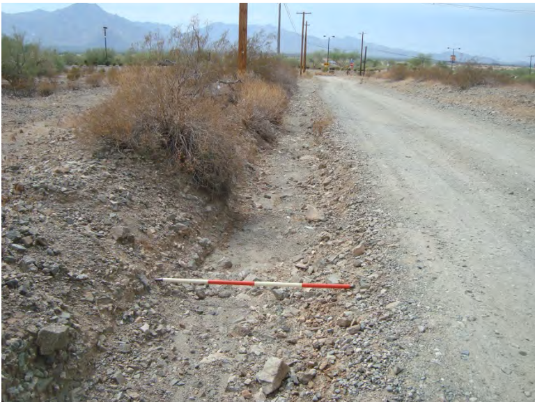
Photo 207. Wash 40 (W40) facing west (downstream); water flows along road ditch; 4-foot-long scale
