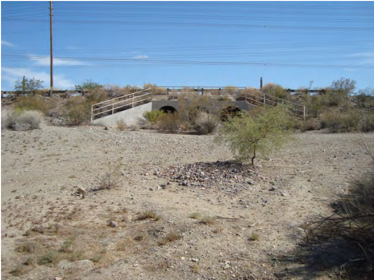
Photo 47. Detention basin (DB) near outlet facing south (downstream) to Pecos Road; no channel to outlet
