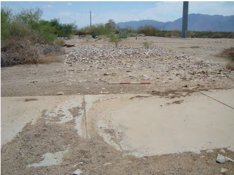
Photo 111. Stormwater feature (SF) conveying drainage from housing development facing south (downstream); water ponds in this location; 4-foot-long scale
