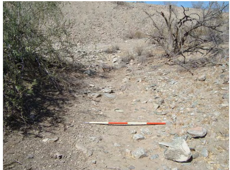
Photo 52. Truncated wash (T1) east of 17 th Avenue facing northeast (upstream); 4-foot-long scale
