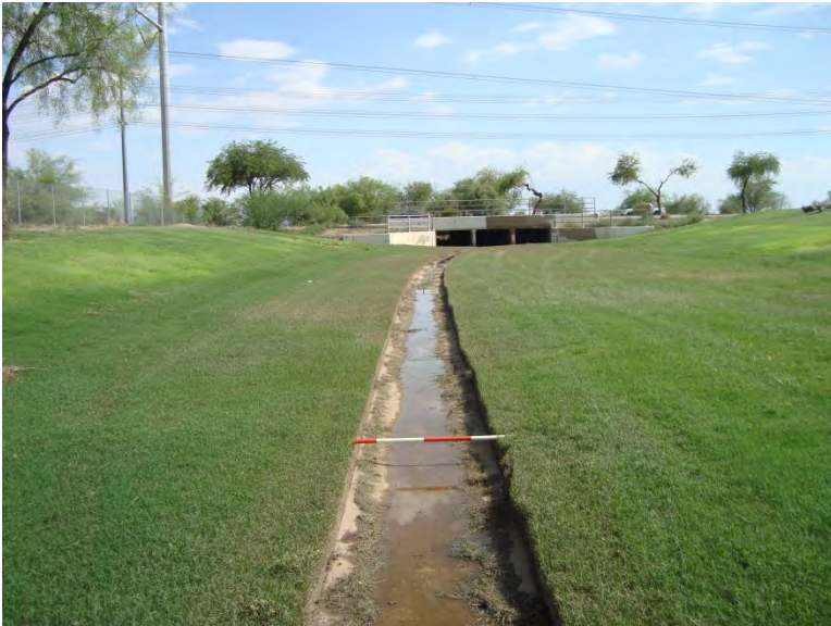
Photo 5. Constructed channel 1 (C1) facing south (downstream) toward Pecos Road; OHWM at the break of slope; 4-foot-long scale
