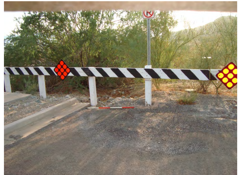
Photo 112. Wash 16 (W16) facing west (downstream) at point where roadway runoff from Chandler Blvd. enters wash; 4-foot-long scale
