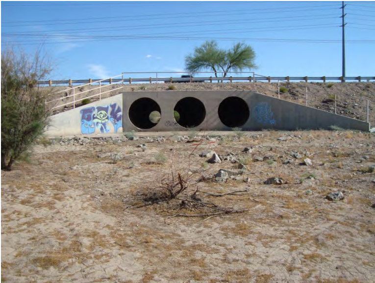
Photo 36. Wash 3 (W3) facing south (downstream) to Pecos Road; 4-foot-long scale near culvert
