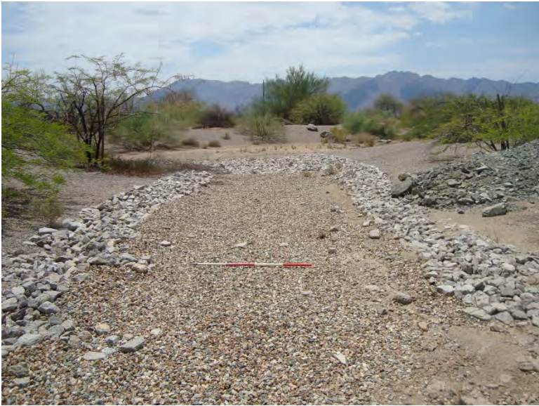
Photo 109. Constructed channel 7 (C7) facing south (downstream) at outlet to detention basin; 4-foot-long scale
