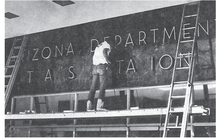
A workman affixes letters spelling out Arizona Department of Transportation on the Administration Building on 17th Avenue in this photo, which originally appeared in the July 1975 issue of Newsbeat, ADOT’s employee newsletter at the time.
