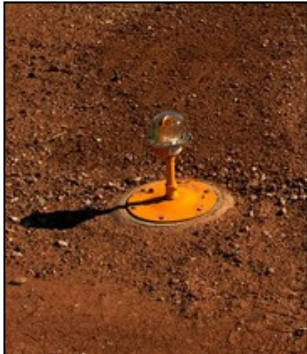
FIGURE 3-3 EXISTING MEDIUM INTENSITY RUNWAY LIGHT
