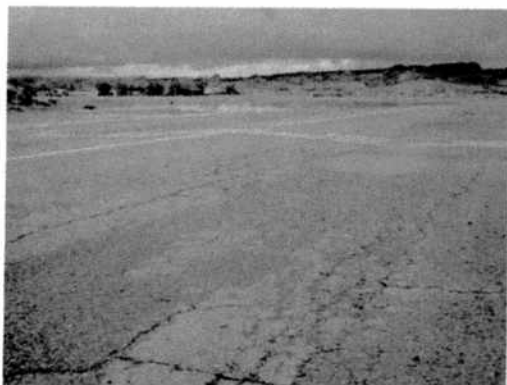
TAXIWAY PAVEMENT SURFACE (NOTE RUTTING)
