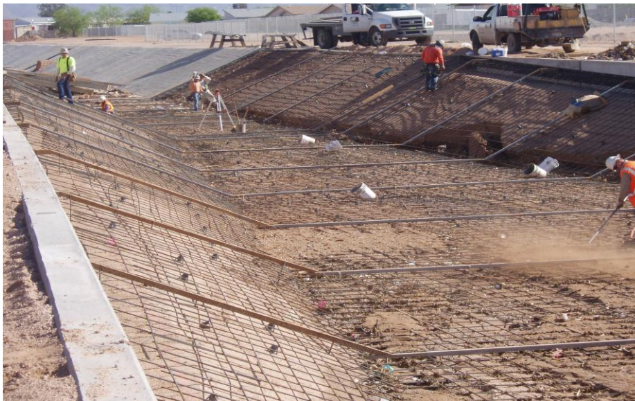
Figure 5. Cleanup Operation for a Canal during Construction When an Occasional Rainfall Results in Debris Accumulation and Grade Changes of the Prepared Base. Photo Courtesy of Rich Shelly, Pulice Construction Co.
