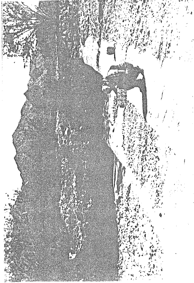
DAMAGE @ SOUTH END OF CHECK WALL (ADOT Bridge Inspection Files)
