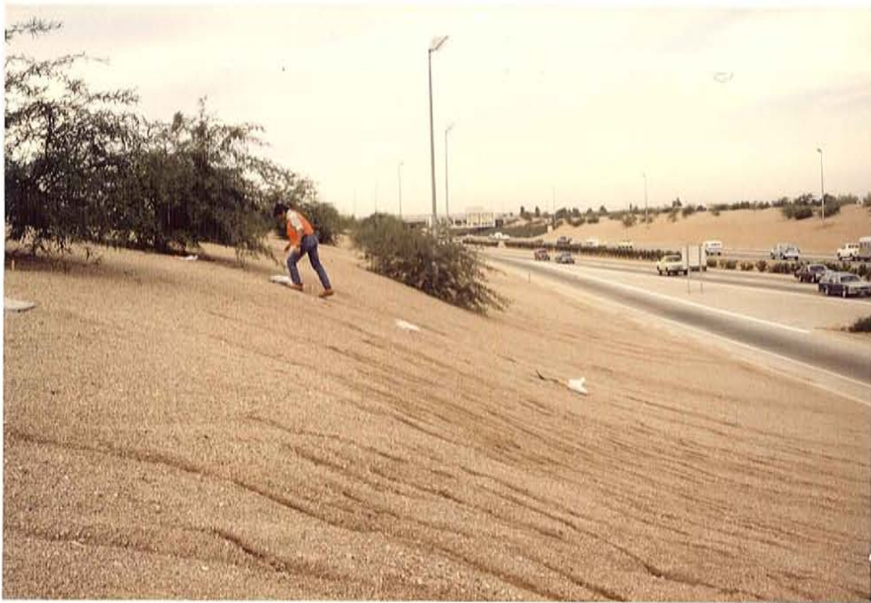
Plate 1. Rock slope protection damage on SR 360 by storm of October, 1987
