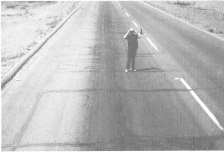
March 25, 1971 23.1% Cracking Before Overlay
