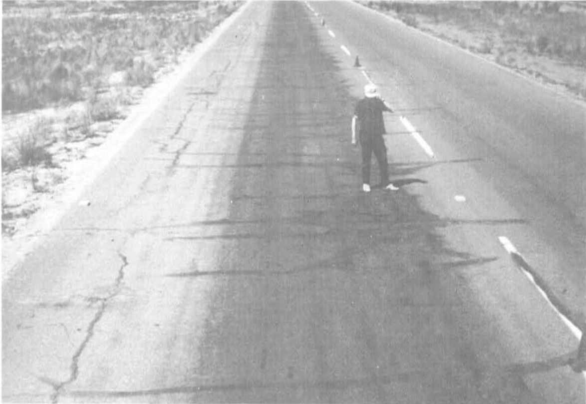
March 25, 1971, 23.1% Cracking Before Overlay
