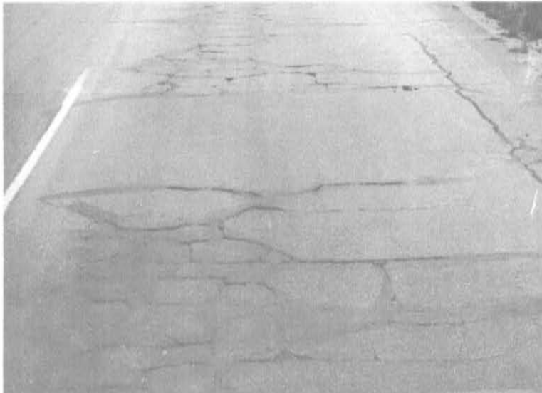
March 24, 1972 31.1% Cracking Before Overlay
