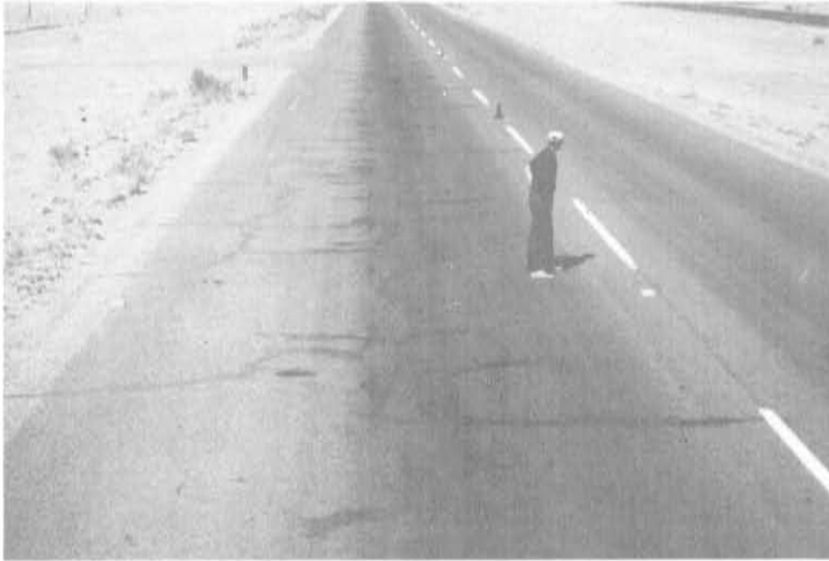
March 25, 1971 13.8% Cracking Before Overlay
