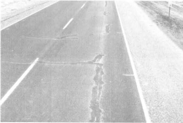
March 13, 1975 8.7% Cracking or 36.7% Reflected Cracking After Overlay
