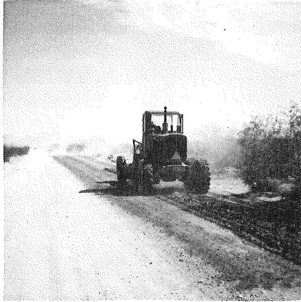
FIGURE 10: ROAD SURFACE RIPPING
