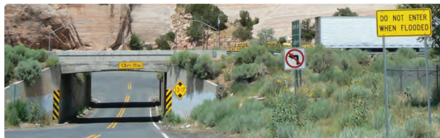
Additional inlets can be installed at the TIs and tied into the existing storm drain system to mitigate the current flooding issues.
