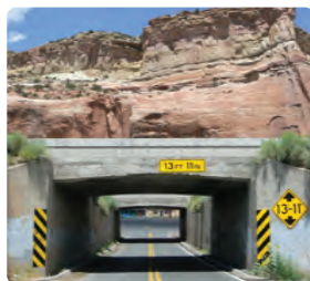
The area's intact sandstone and siltstone will likely provide excellent support for bridge foundations.
