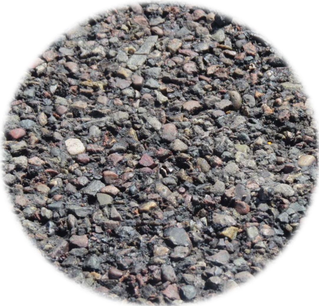
AR-ACFC Rating Unacceptable Pavement
