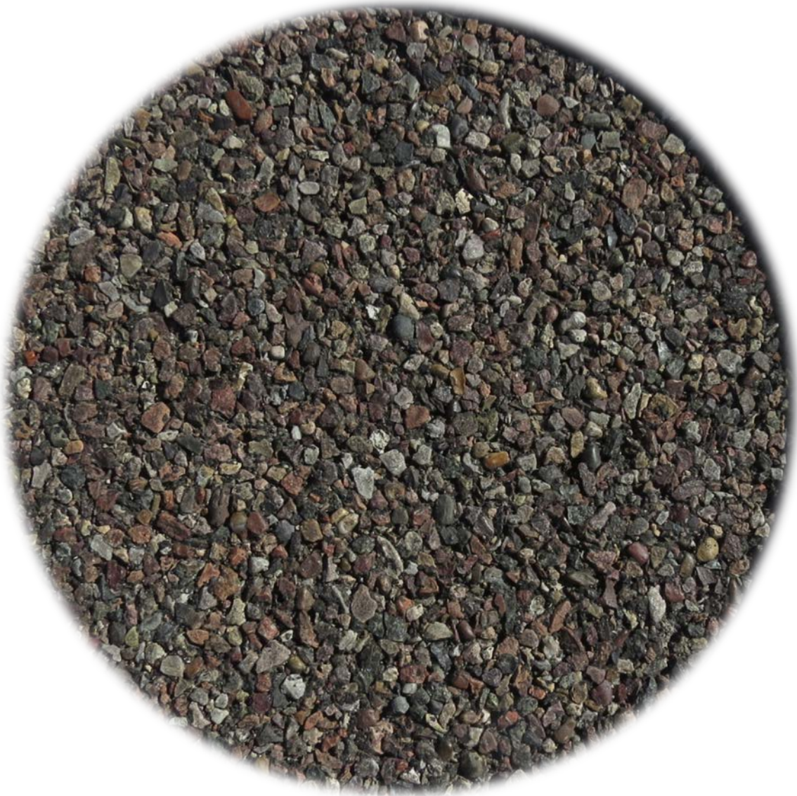
AR-ACFC Rating Good Pavement
