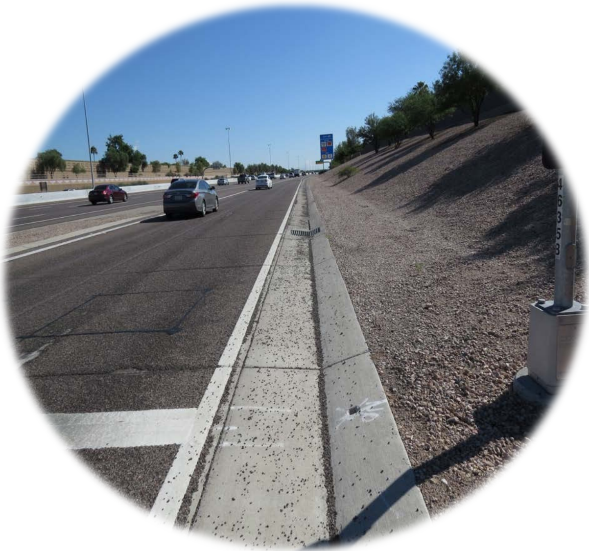
Material accumulation outside of travel lanes (Unacceptable)
