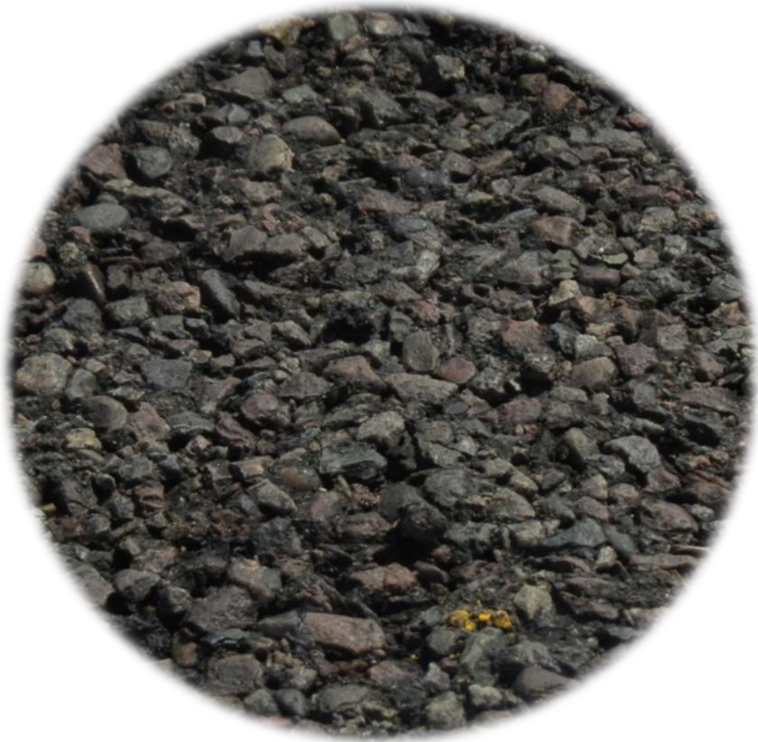
AR-ACFC Rating Unacceptable Pavement
