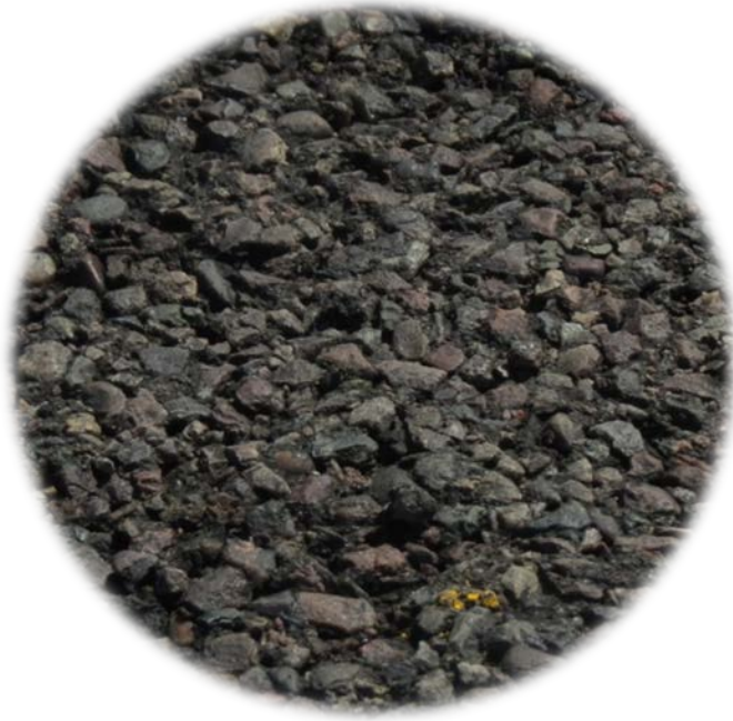
AR-ACFC Rating Unacceptable Pavement
