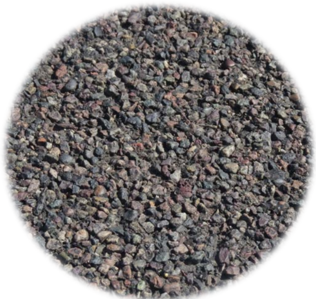
AR-ACFC Rating Unacceptable Pavement
