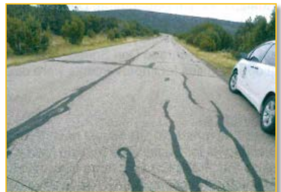
Pavement conditions along Supai Road (BIA 18) were cited as a major safety issues in the 2011 BIA 18 Road Safety Assessment Report.
