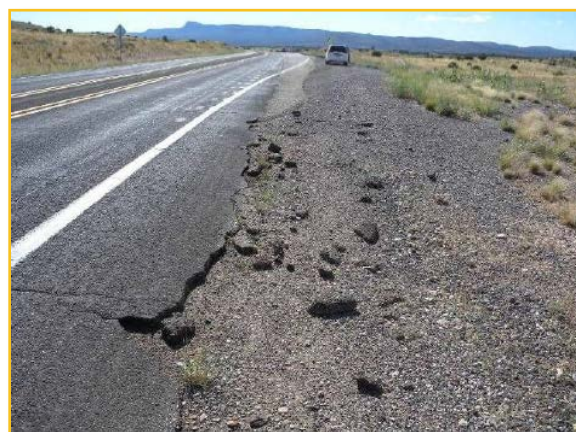
Pavement deterioration was noted along State Highway 66 from MP 96 to 112.3 RSA
