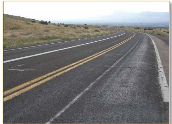
Faded pavement markings identified in the SR 66 MP 96 to 112.3 RSA
